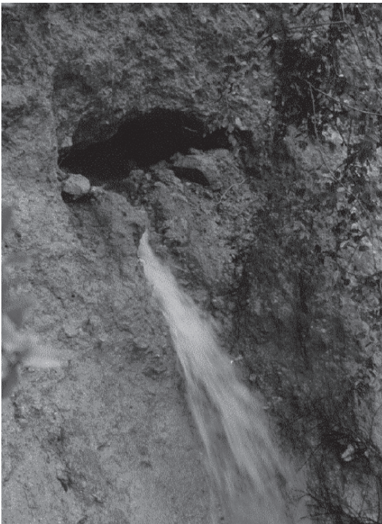
Figure 8. Erosion pipe with heavy seepage
