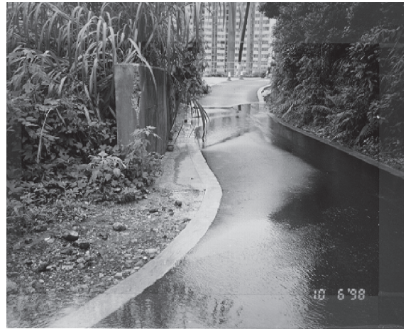
Figure 7. Ponding due to poor surface drainage provision
