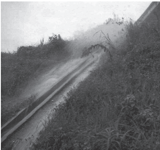
Figure 6. Over-spilling due to inadequate surface drainage detailing
